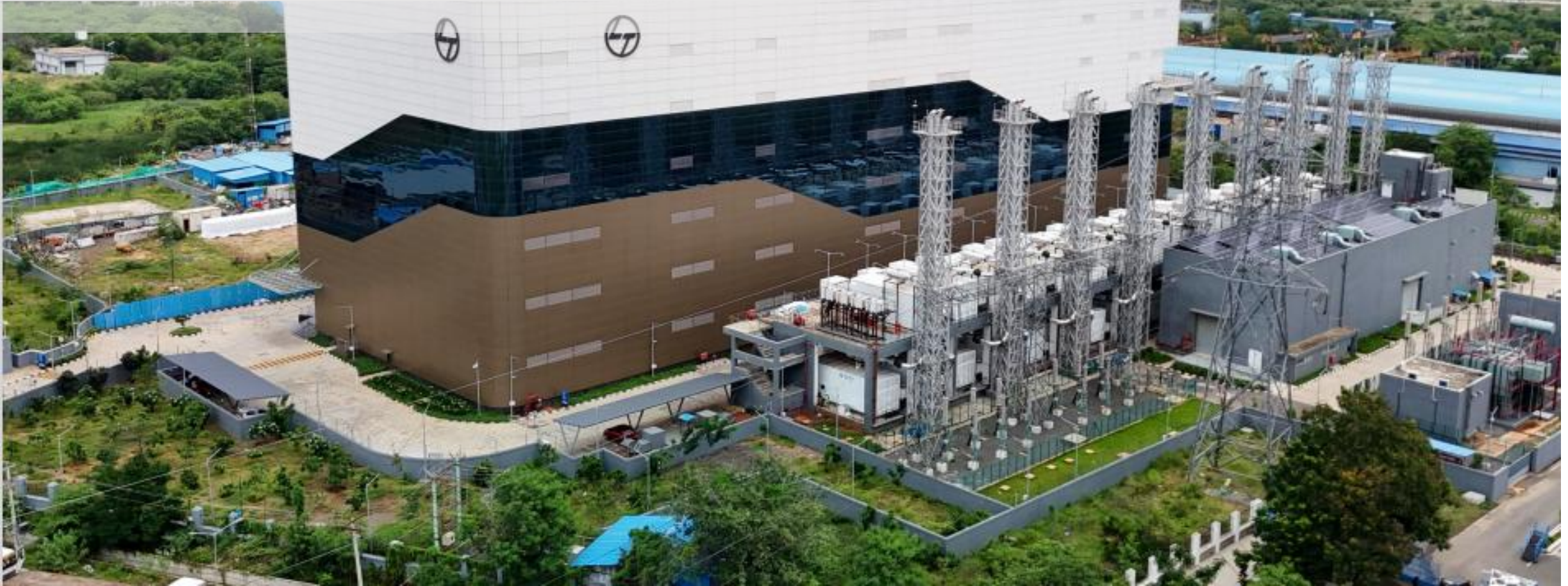
L&T Data Center, Sriperumbudur, Tamil Nadu
